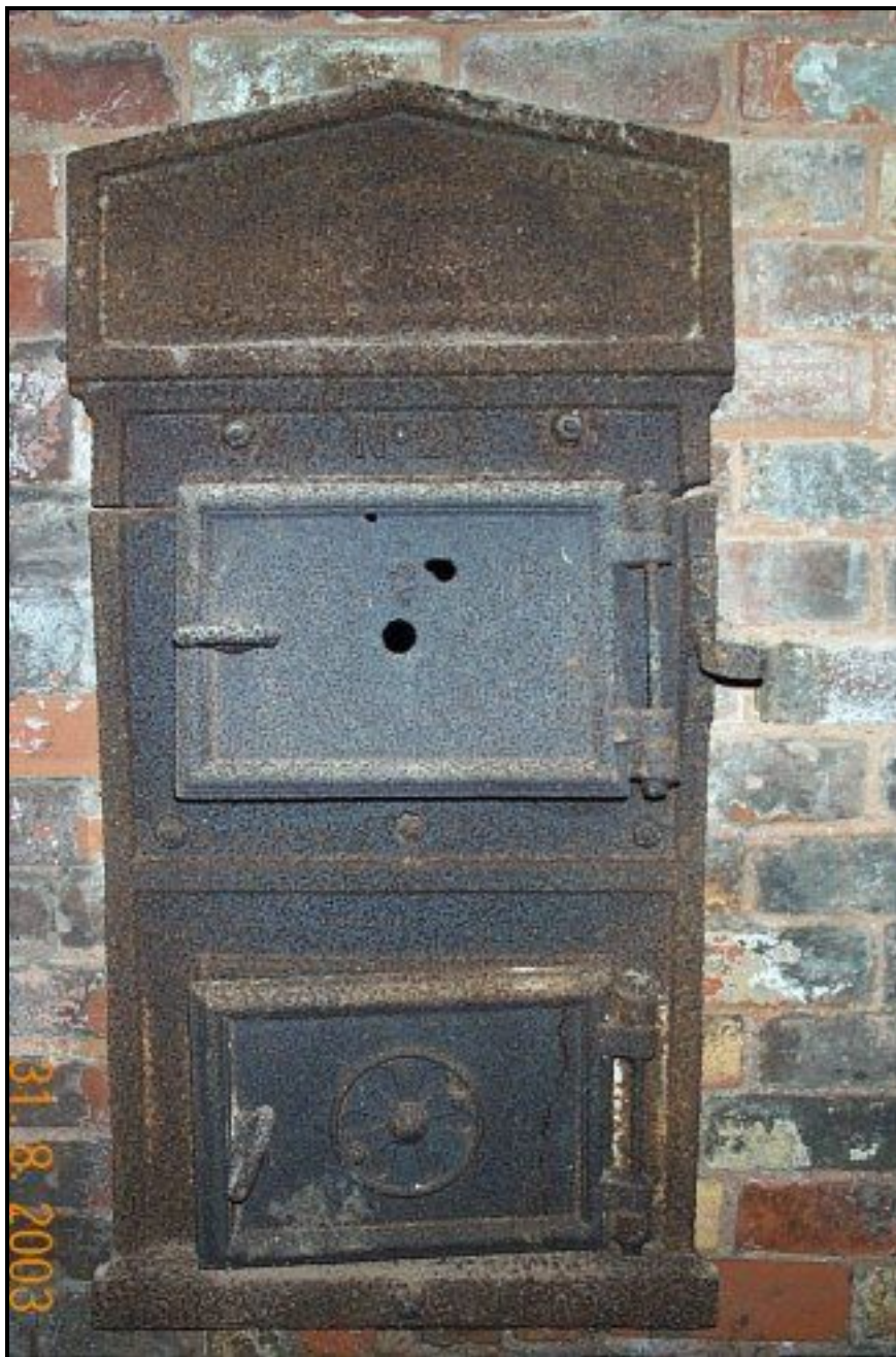
Haden stove at St Mary the Virgin, Hanbury, Worcestershire
